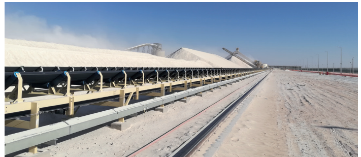
High speed overland conveyor
